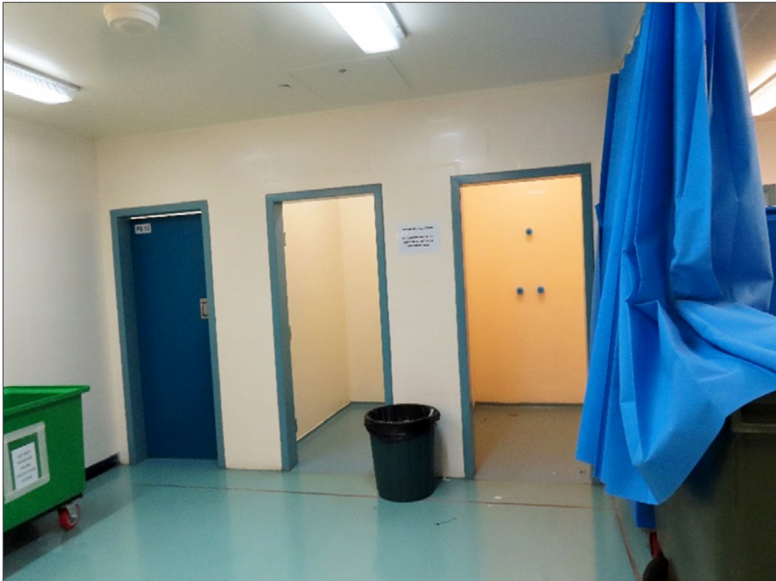
Photo 1: Two non-operational shower cubicles in the reception store
