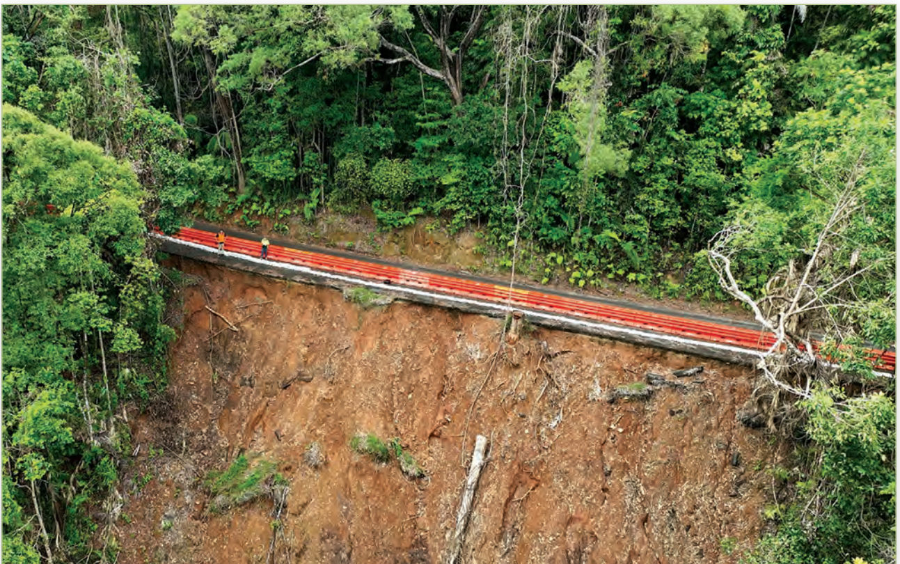
Impacts to road infrastructure and surrounding forest after TC Jasper. Alexandra Range, Eastern Kuku Yalanji Country—Wet Tropics Images
