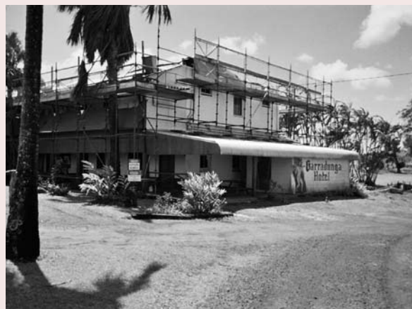
Repair work is still in progress following the devastation of Cyclone Larry
