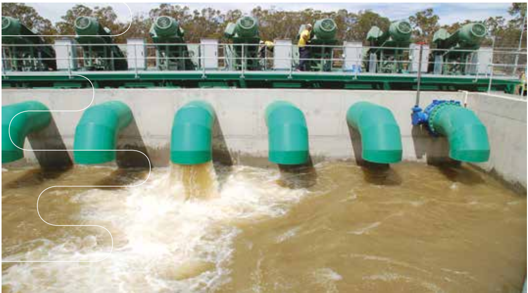
The Hattah Lakes water management structures include large pumps to help bring water from the River Murray into the lakes system (photo by Heather Peachey, MDBA).
