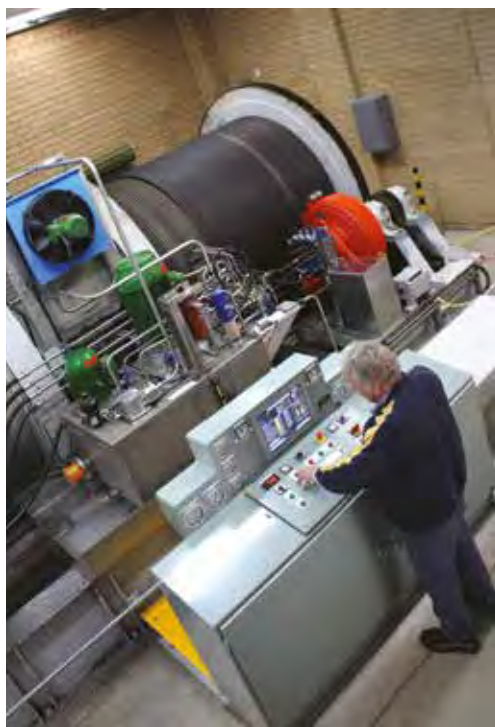
Dartmouth senior reservoir controller Peter Liepkalns demonstrating the newly completed low level outlet winch drive system. The winch raises and lowers the low level bulkhead, which weighs 25 tonnes. It is lowered to close off the reservoir's outlet tunnel so that inspections and maintenance can be carried out (photo by Andrew Beer, MDBA).
