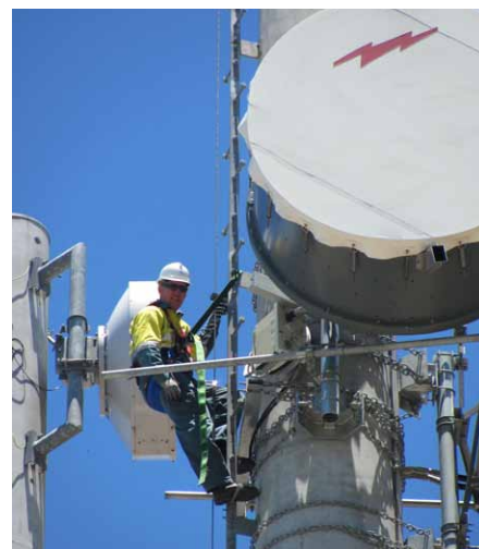
Ergon Energy is rolling out an all-encompassing telecommunications network, known as 'UbiNet', that will link 40 of our depots and 90 substations, including the Bundaberg substation site where Installation Deliver Manager Wayne Carr is inspecting the installation of the new telecommunications equipment.
