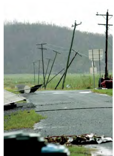
The response saw around 600 kilometres of electricity cable and conductor line and almost 2,300 poles and cross arms brought in to rebuild lines like this one near Tully – as well as around 25,000 fuses, 6,700 insulators and 350,000 bolts, screws, brackets and clamps.
